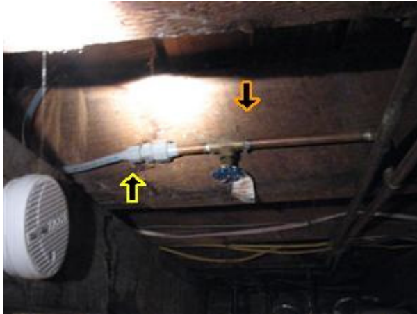
6.1 Picture 1 Poly pipe and on the right is the leak.
