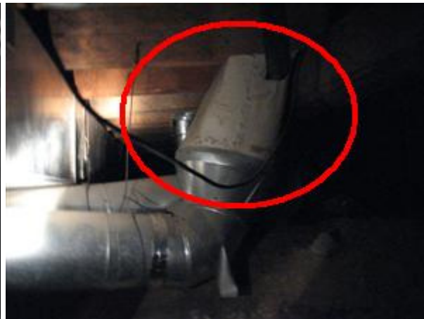
8.3 Picture 2 One example of asbestos like duct compent
