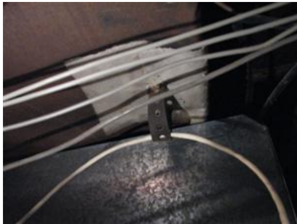
8.3 Picture 1 Asbestos like tape
