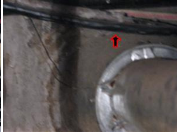
7.3 Picture 2 100 amp cable resting on exhaust furnace pipe collar
