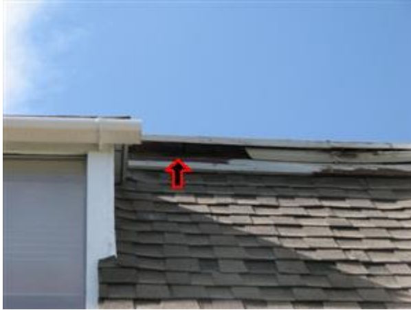
2.4 Picture 1 Missing piece of fascia board
