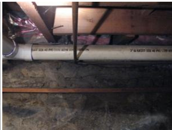
6.3 Picture 2 Pipes resting on top of each other
