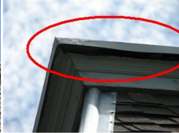
2.4 Picture 2 Typical fascia deterioration
